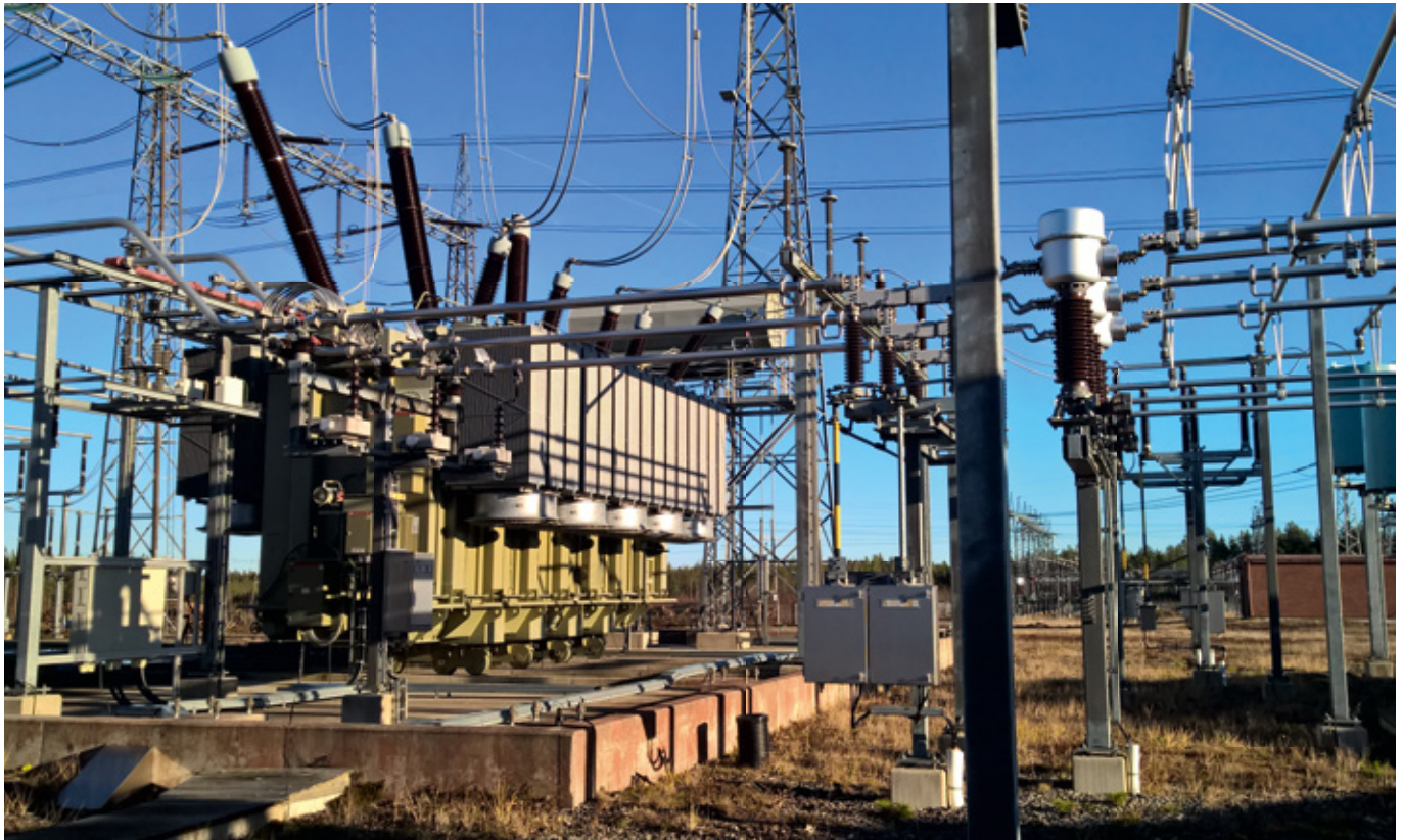
The Optimus DGA Monitor is the right solution for safe guarding critical transformers in harsh environments
